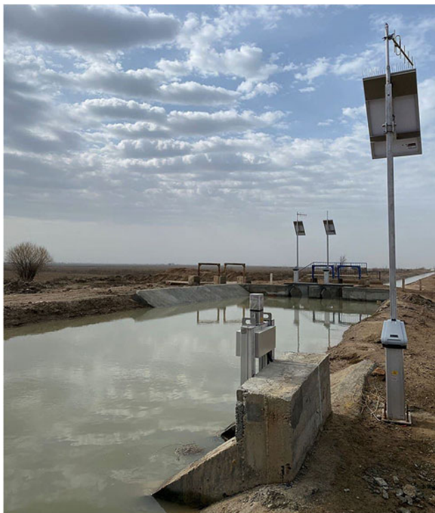
Fig. 7 Introduction of Smart Water system for real-time water control. The Kasbi district of Kashkadarya region, Uzbekistan
