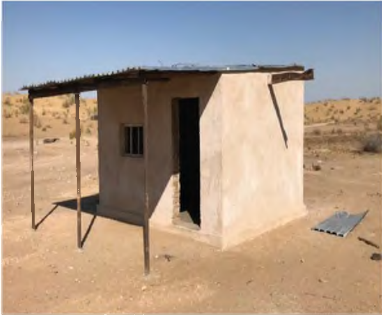
B) Renovated house, allowing shepherds to stay in the pastures for two additional seasons (after project implementation)
