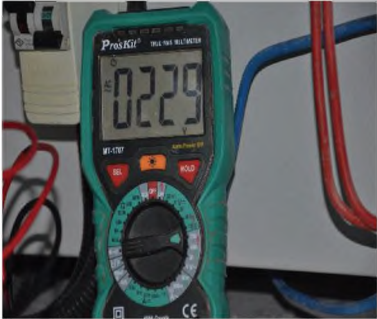
E) Solar generated electricity is on
