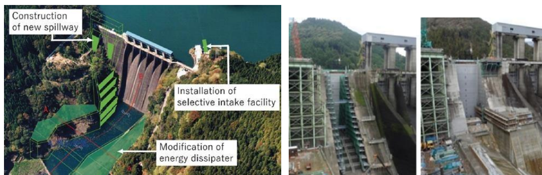
Figure 5-15 Example of intake and discharge facilities modification at Nagayasuguchi dam (Sasaki and Kondo, 2018)
