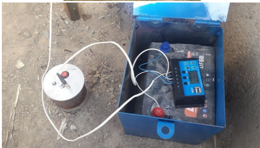
Picture-2. Smart meter in monitoring well
